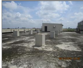
Photo of fire safety equipment Rooftop.JPG
