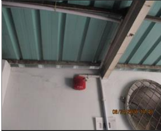
Photo of fire safety equipment Fire Alarm.JPG
