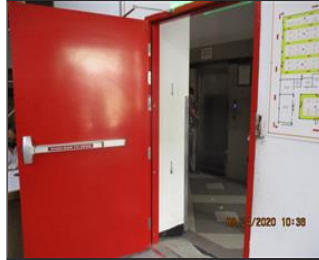
Photo of fire safety equipment Fire Door.JPG
