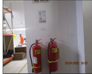
Photo of fire safety equipment Fire Extinguisher.JPG
