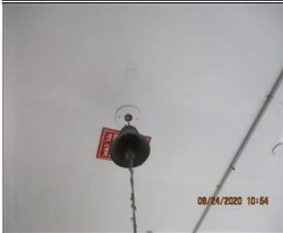
Photo of fire safety equipment Gong Bell.JPG
