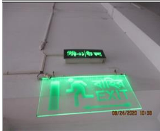
Photo of fire safety equipment Exit Sign.JPG
