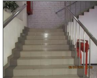
Photo of fire safety equipment Stair.JPG
