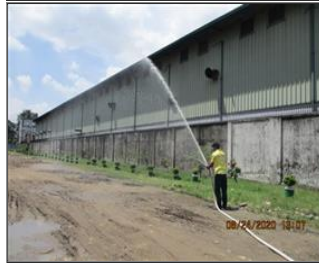
Photo of fire safety equipment Fire Hose Pipe test.JPG
